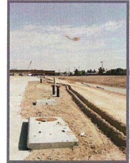
Target, Loop 375 Front-Curb Inlet Cap, Back- PSB Valve Box
