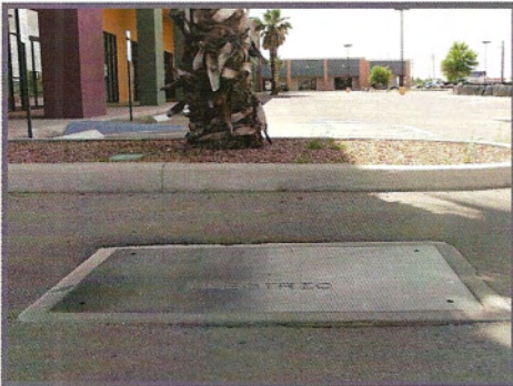
El Paso Electric Traffic Bearing Box, Downtown Horizon Plaza
