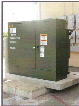
Downtown Horizon Plaza , Electrical Pedestal
