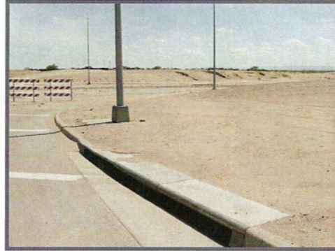
Loop 375 & East Lake, Curb Inlet
