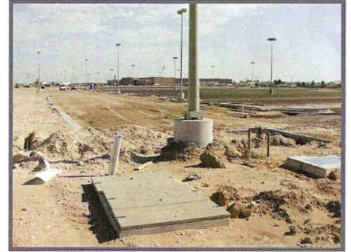
Target , Loop 375 Electrical Boxes
