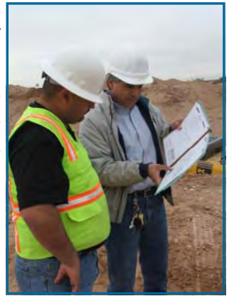
John Franklin of WPCI talks with Emilio Gonzalez regarding the upcoming installation
