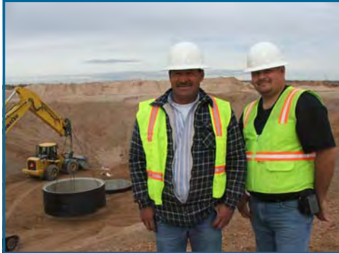
Luis Diaz and Emilio Gonzalez, Redcliff Project Superintendents at Tres Sueños lift station site
