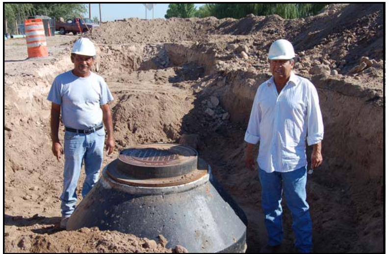
Pablo Ramos, Site Manager and Pedro Hernandez of Southwest Growth Stand next to recent manhole install in San Elizario,,
