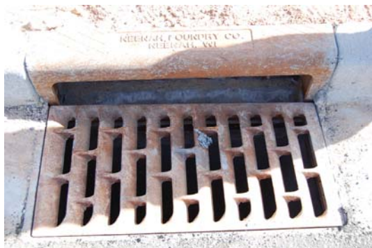
Inlet installed at Lowes site for water drainage in the parking lot.
