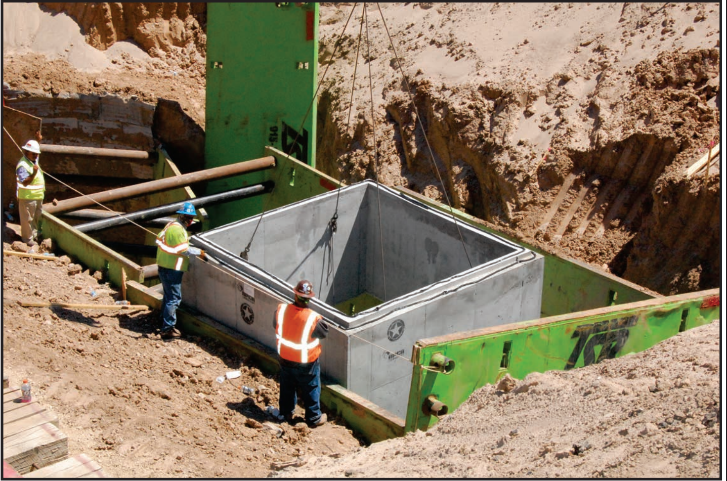
10 x 10 ID custom structure by Western Precast being set at CMD's job site.
